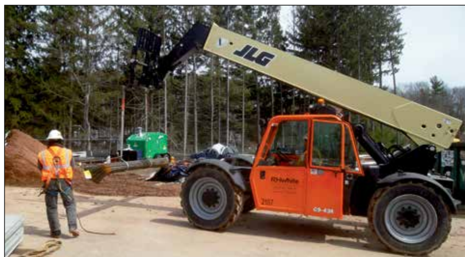
A JLG G9-43A Telehandler transports a bundle of rebar to a concrete slab construction area.
