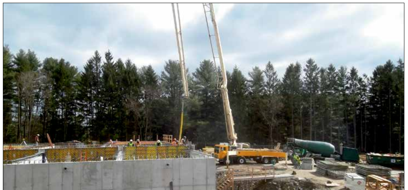
Modern Concrete Pumping's 45-meter Schwing delivers ready mix from Builders Concrete East transit mixer to crews placing tank walls.
