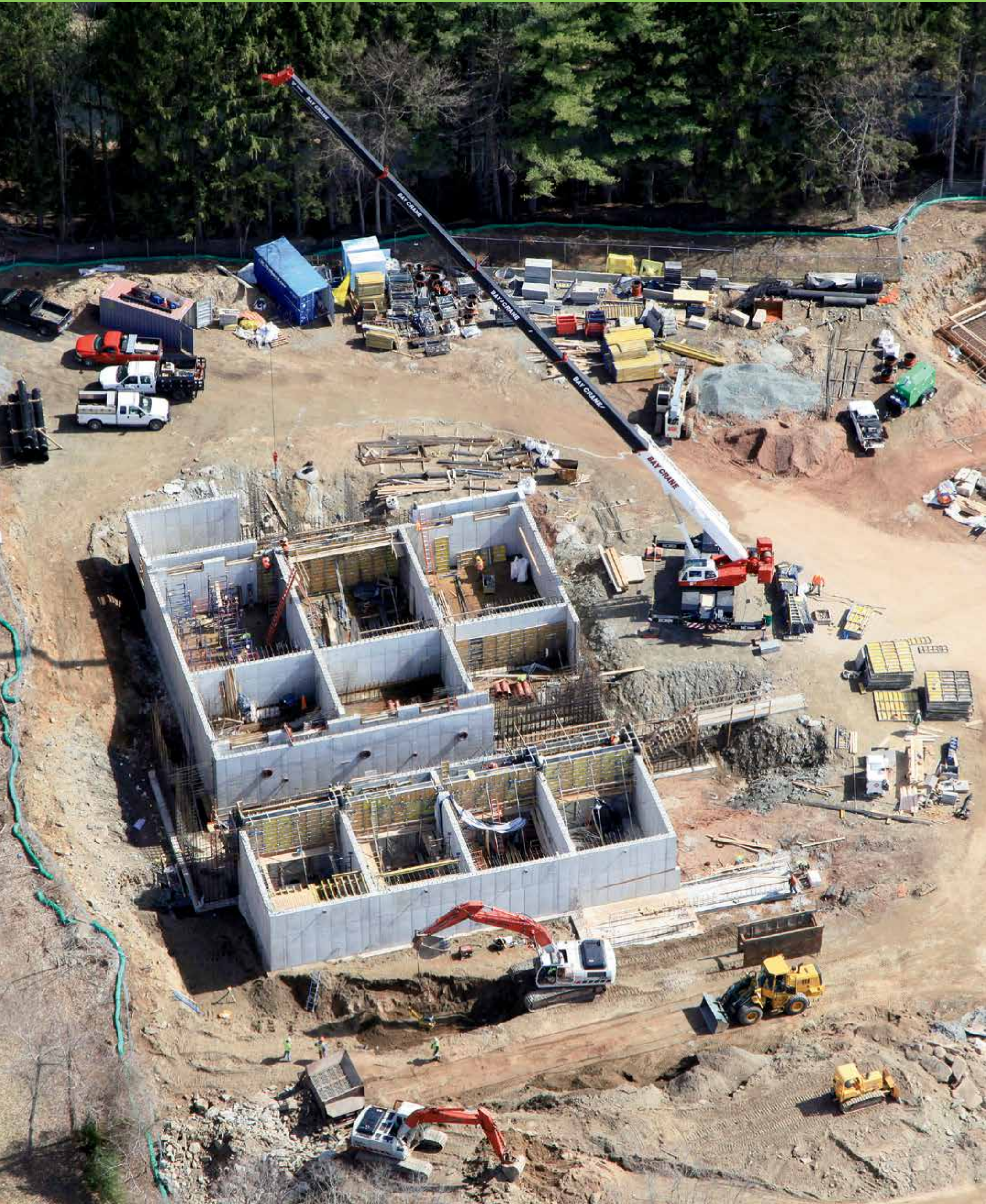
Aerial view shows hydraulic Bay Crane passing materials to crews inside DAF tanks of new building, while at right is partially built Spent Washwater Tank.
