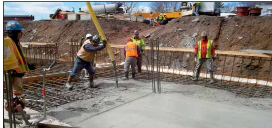
Ready mix is placed for floor slab by HOP River crew, which is responsible for forming and placing about 4,000 cubic yards of concrete for the job.
