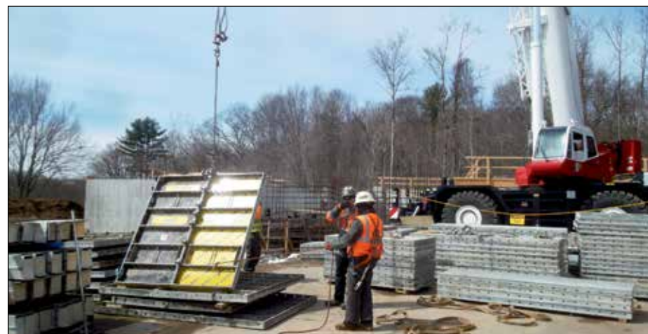
Bay Crane hoists a Doka Frami Xlife concrete form for tank wall pour.
